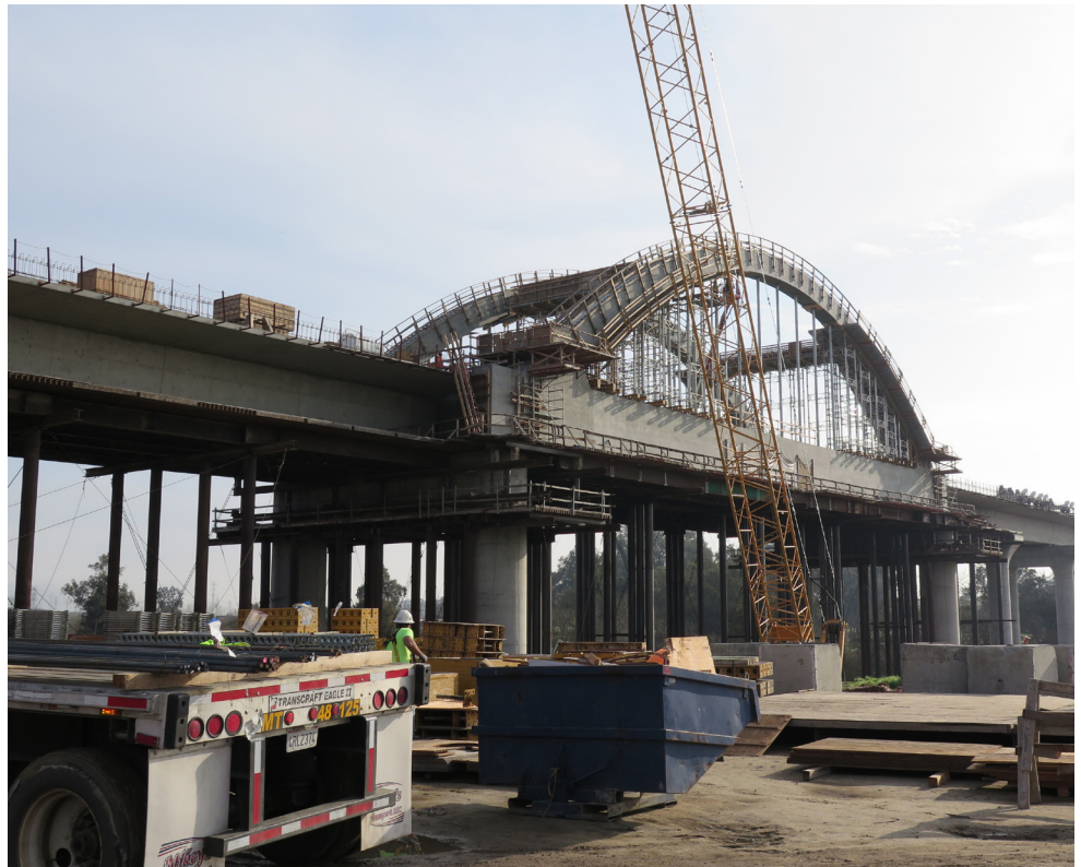
California High-Speed Rail San Joaquin River Viaduct under construction in 2020 – photo from CAHSRA
